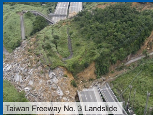
Taiwan Freeway No. 3 Landslide
